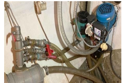
Deep freeze and fridge pumps
