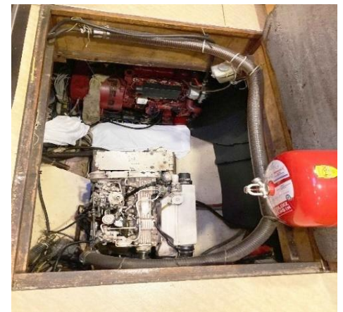
Perkins engine and generator 2
