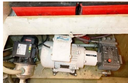
Water maker pumps
