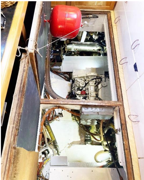
Port engine room
