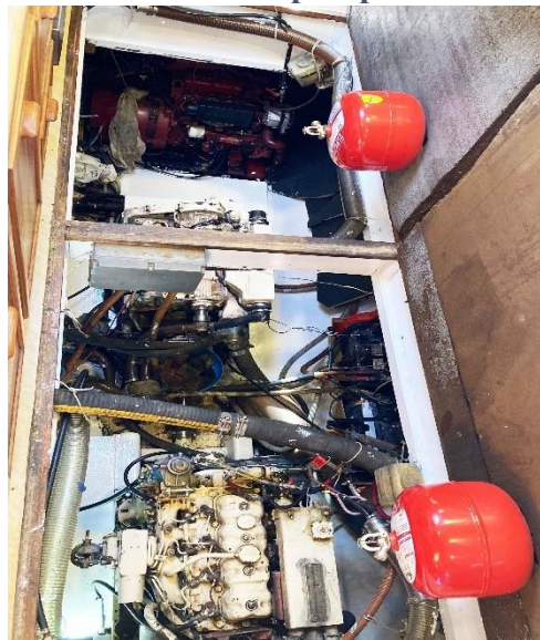
Starboard engine room
